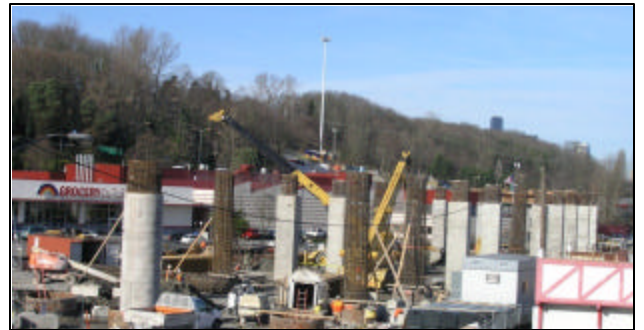
Pouring concrete for the elevated trackway (above) Constructing columns for the Mount Baker Station (below)
