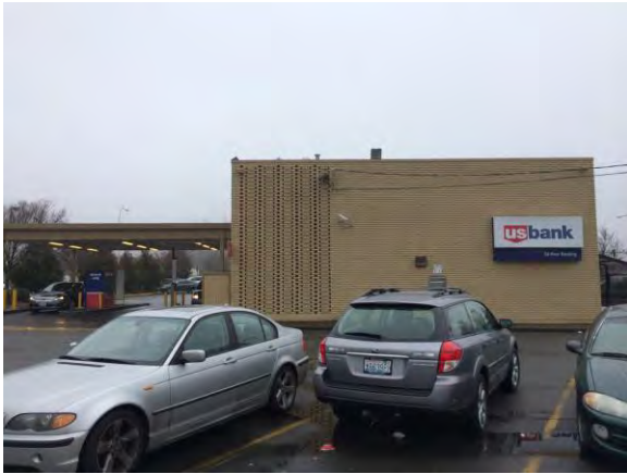
Single section of honeycomb brick is visible at left side of wall. West elevation 2013
