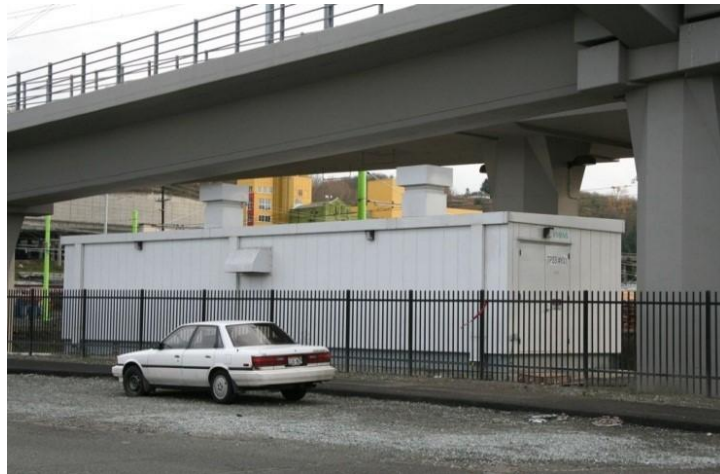
Figure B3-5 Traction Power Substation
