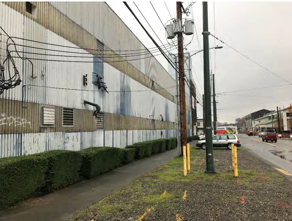
Photo 4. Subject property, looking east. Pole-mounted transformers adjacent to the building.
