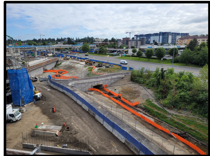
Scriber Creek Daylit in Lynnwood Adjacent to Parking Garage and Transit Center
