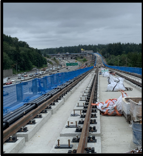
Direct Fixation Trackwork on Elevated Guideway in Seattle
