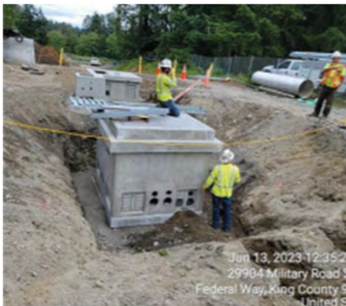
PSE Power Vault Installation at Military Rd in Federal Way
