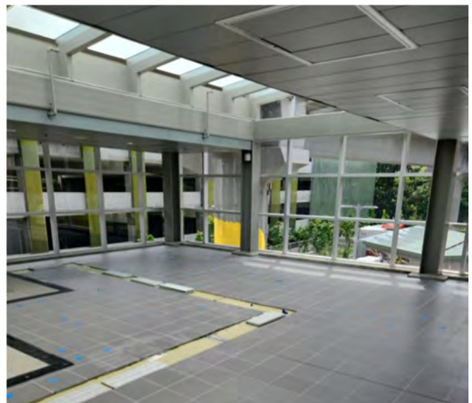
Damaged south mezzanine tiles to be replaced
