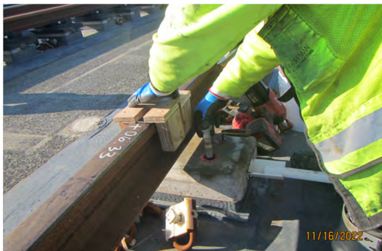
E130 Seattle to South Bellevue: Installing new nylon inserts, westbound on the floating bridge
