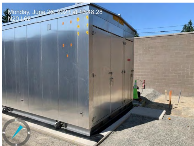
Signal House delivered and set in Mountlake Terrace
