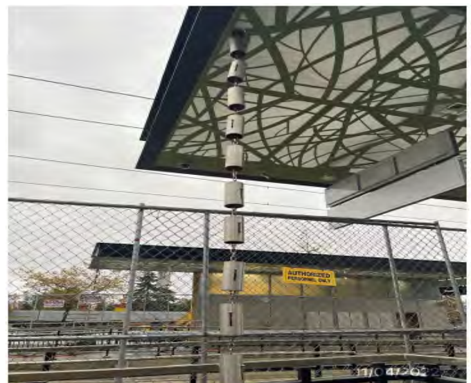
Rain Chain at 130th Station Repaired and Closed off the Punch List.
