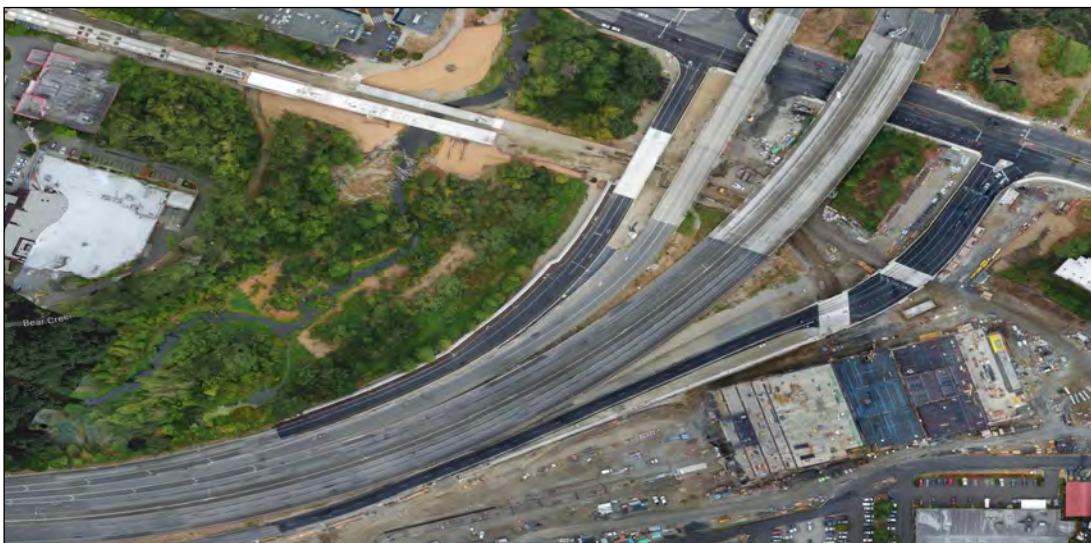
Artist Rendering of Marymoor Station (above) and Bird's-eye View Current Progress (below)
