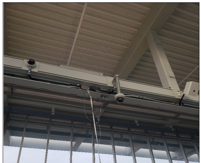
Camera installation at Northgate Station.
