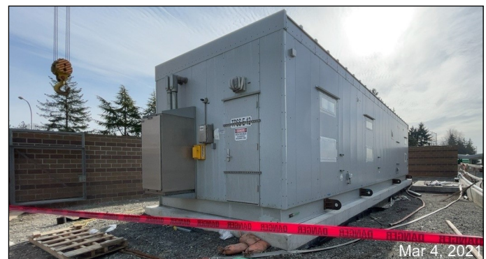
TPSS unit delivered and set in-between East Main Station and Bellevue Transit Center Station.
