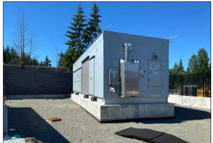
Representative Traction Power Substation (TPSS) Unit.
