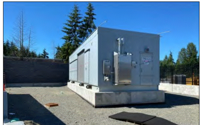
Representative Traction Power Substation (TPSS) Unit.
