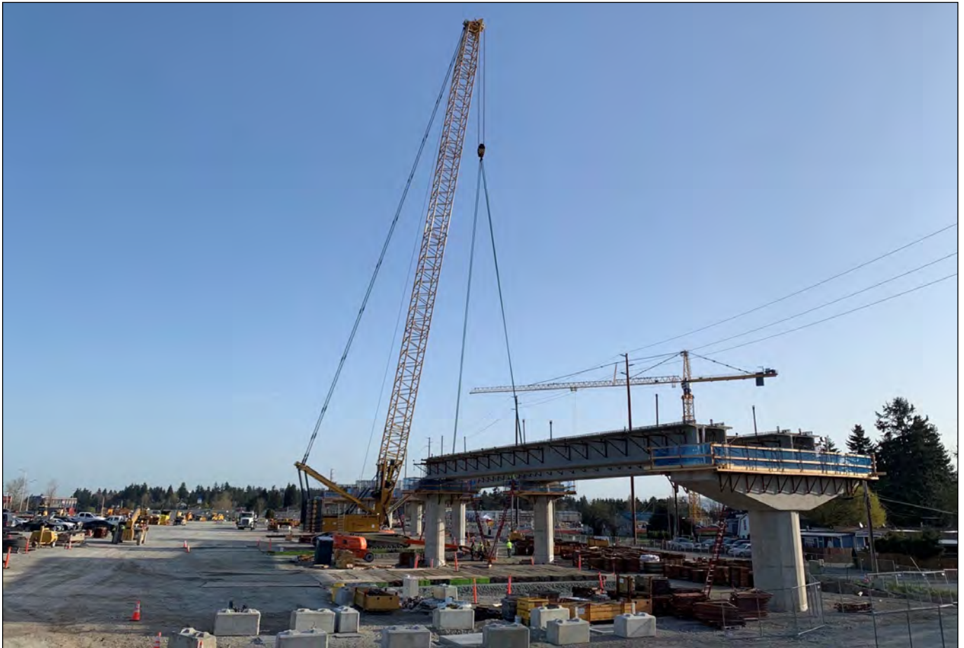
Setting the first girders spanning the columns that form the elevated guideway near the Kent-Des Moines station
