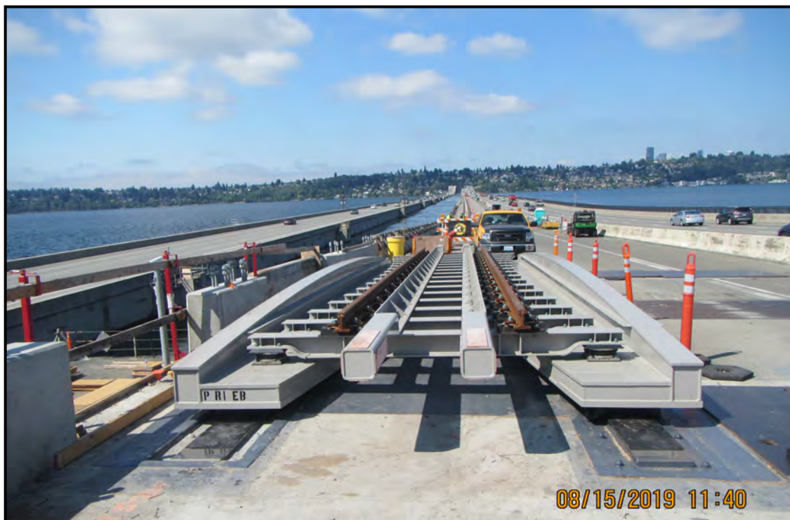
E130 Seattle to South Bellevue: Track Bridge installation on the I-90 floating bridge.
