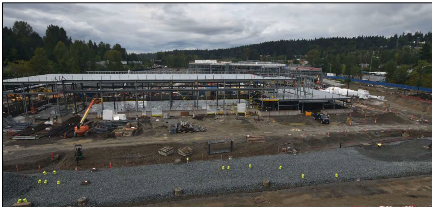
OMF East looking north taking shape with yard scope and steel structure framing on August 30, 2019
