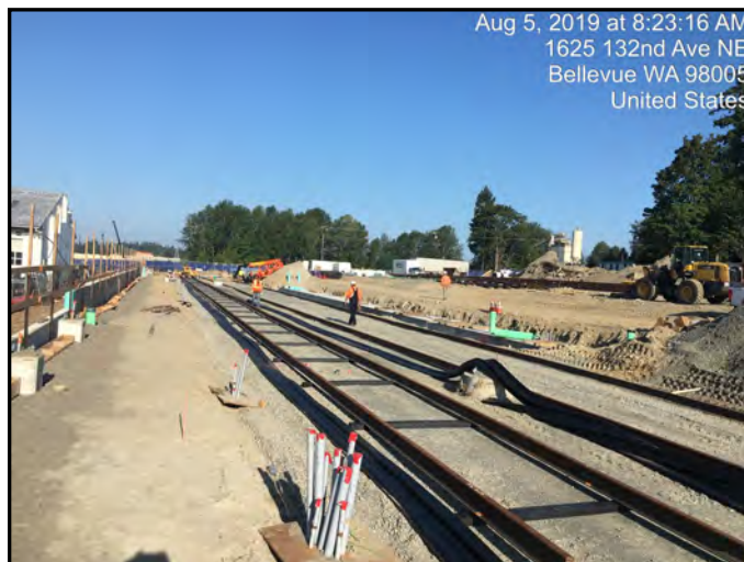
Placing the station rail on the ties and rolled out the boot, looking west.
