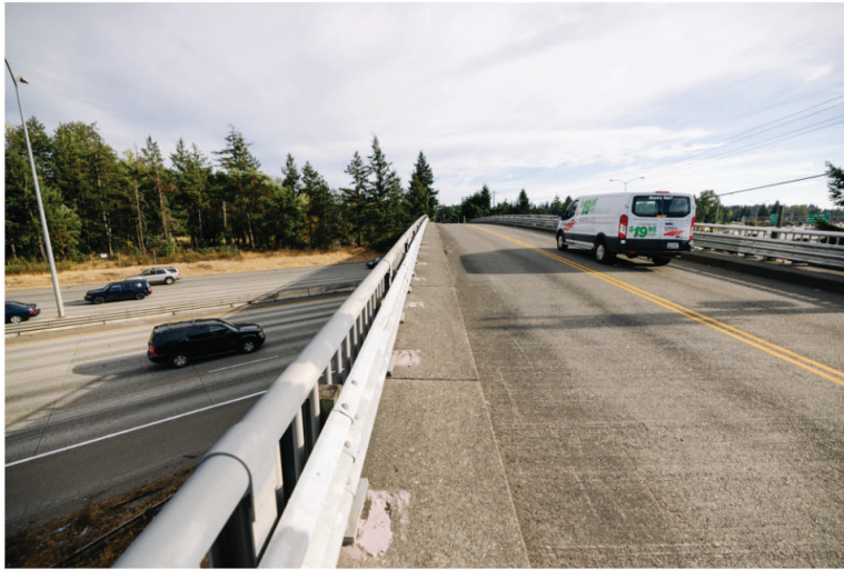
Current view of the 47th Ave SW bridge, seen from the north, with narrow sidewalks on each side.
