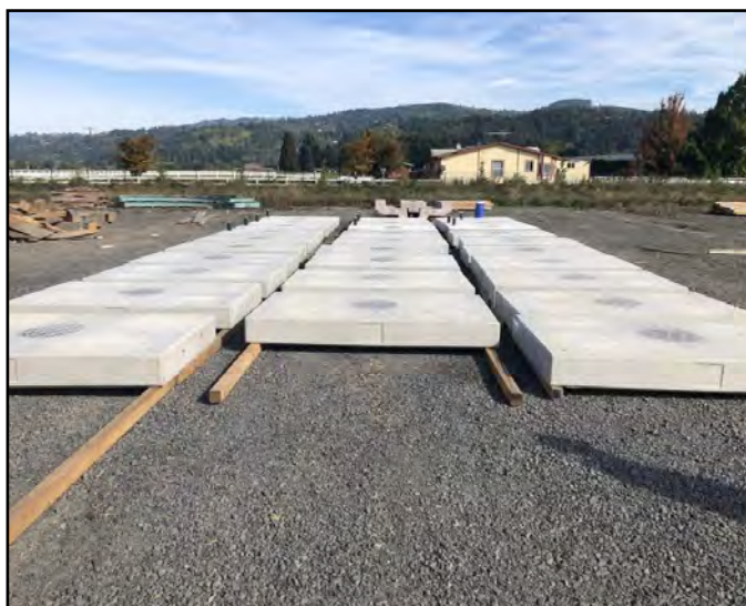
16Hz Floating Slabs from Columbia Precast Products LLC.
