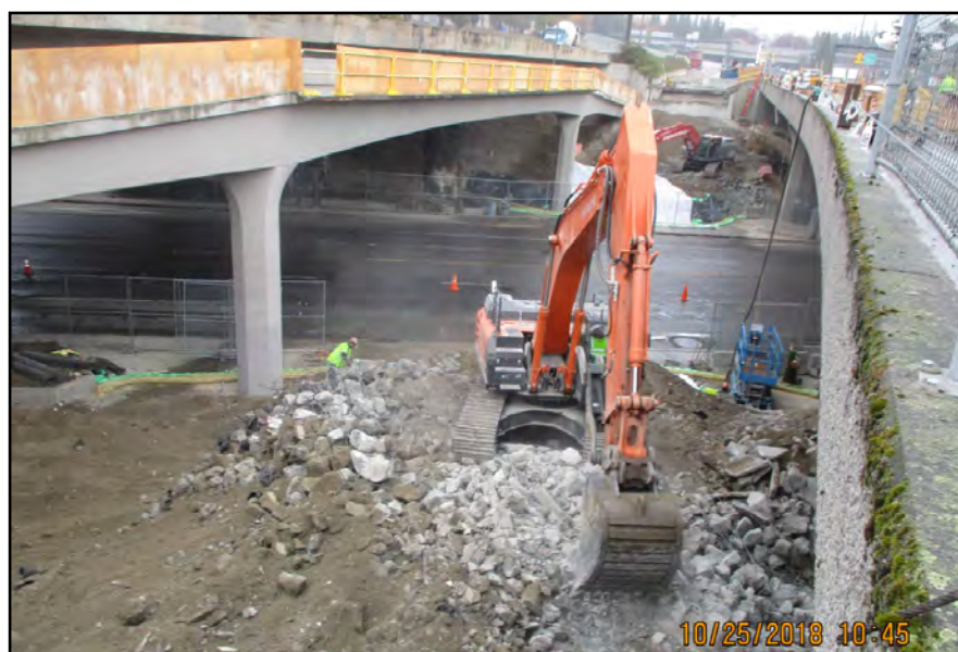
E130 Seattle to South Bellevue: Demolition of access ramp on I-90 along Rainier Ave-
