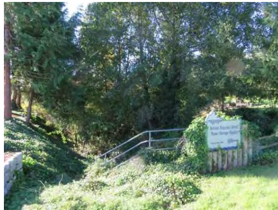
Belmor Mobile Home Park, added stormwater facility
