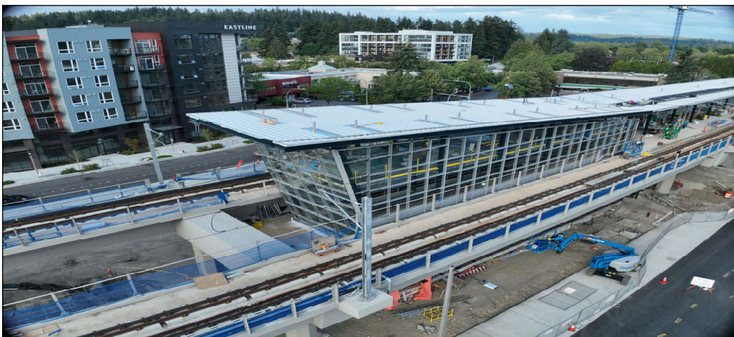
Artist Rendering of Downtown Redmond (above) and Bird's-eye View Current Progress (below)
