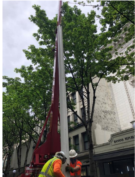
Westlake Pump Test: A drilling rig was located in Downtown for 6 weeks to test groundwater near the future Westlake station. Thank you for your patience as crews completed this important work!
