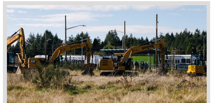
Ready to dig in: Excavators are lined up and ready to go at the Prisma project developed by Bellwether Housing.
