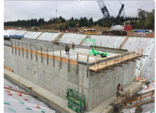
Overlake Village Station Detention Vault
