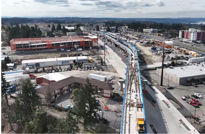
Kent Des Moines Station Direct Fixation Track
