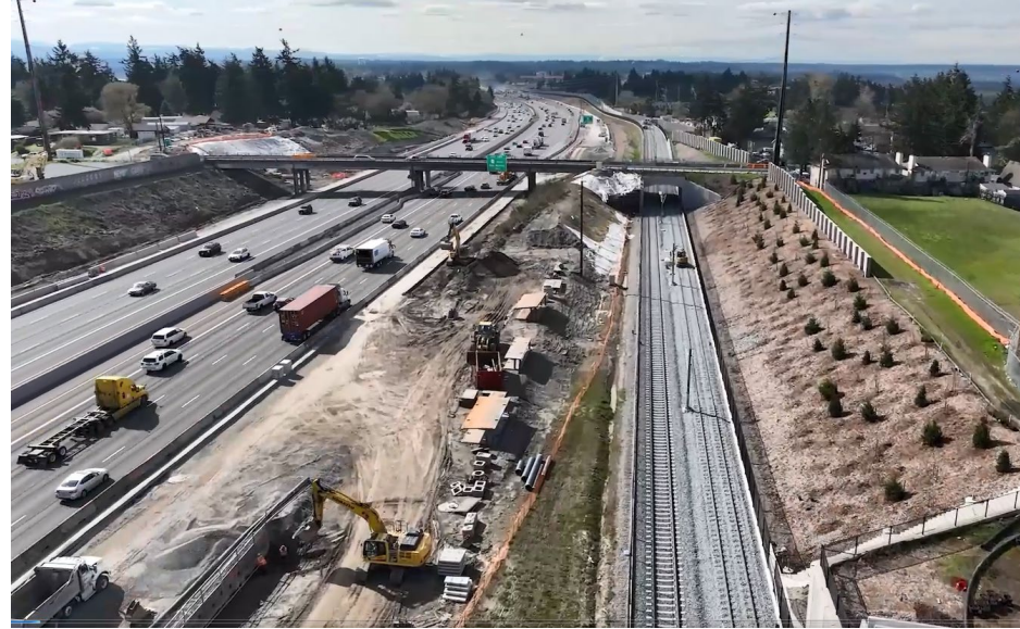
Ballasted Track and Traction Power Poles
